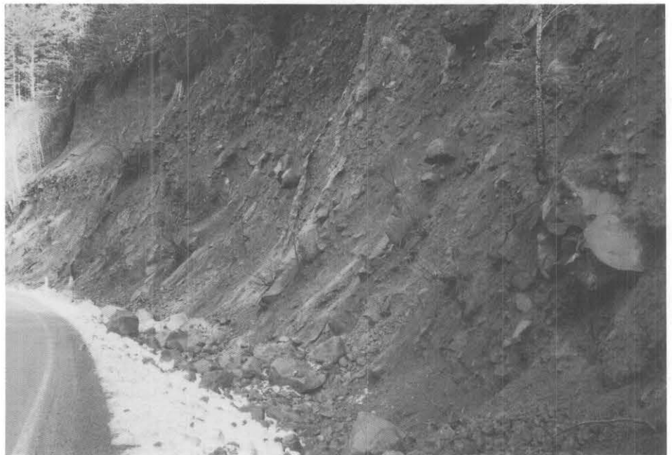
Figure 5.25 Oversteepened soil/rock slope
