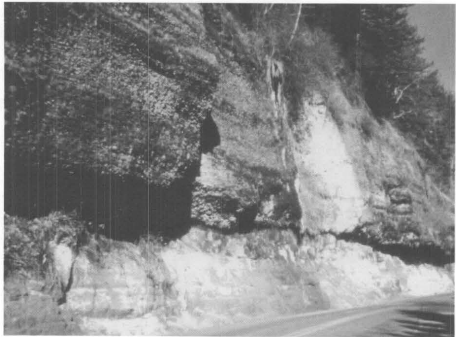
Figure 3.4 Overhanging slope caused by differential erosion.
