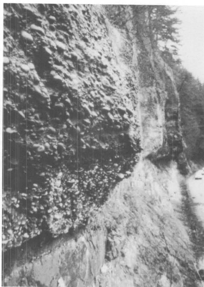
Figure 3.6 Ineffective roadside ditch.
